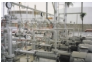
CEH pumps in a carousel filling plant
