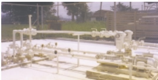
PC plant for automotive refuelling
